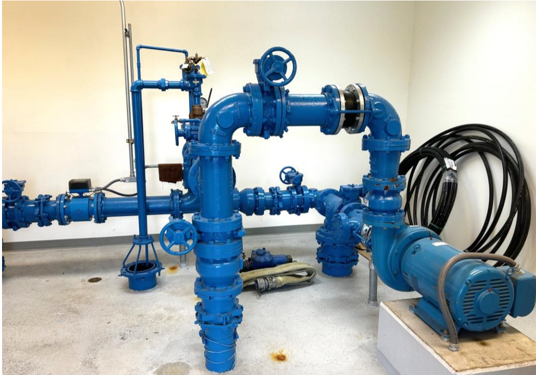
Figure 9 –Booster Pump Station Piping
