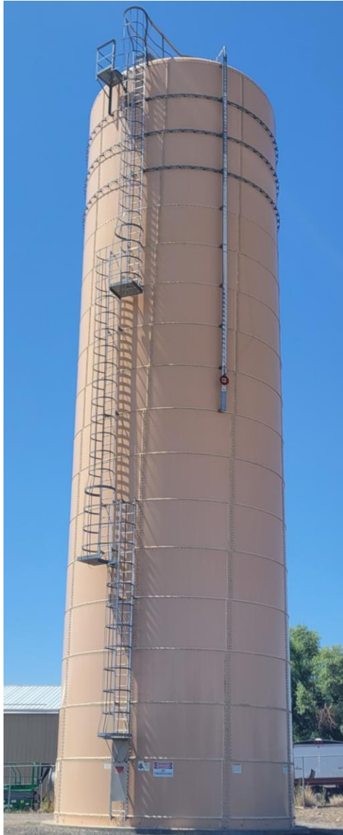
Figure 5: Glass-Coated Steel Bolted Tank Reservoir
