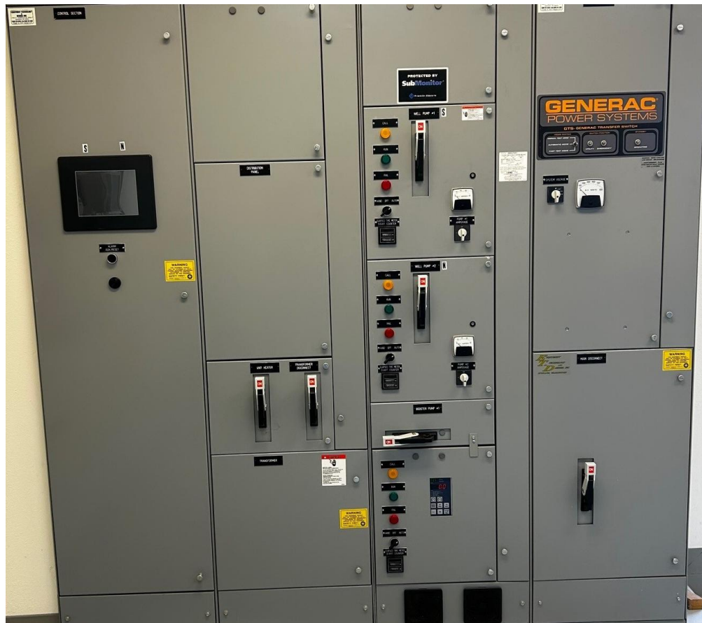
Figure 8 – Booster Pump Station Control Panel
